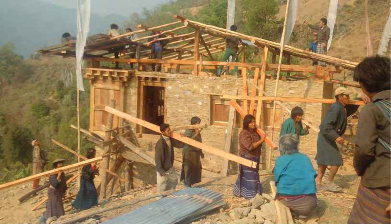
Community members of Dak, Monggar working at the construction of Ap Lekhi's house
