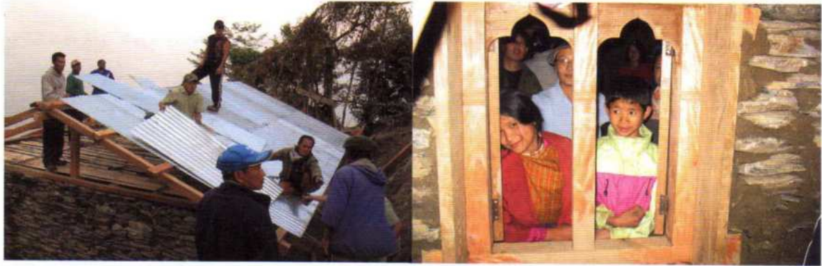
House construction nearing completion on the 3rd day, Lotukuchu, Samtse. Gzey Lham and her brother Sonam Tshering in their new house.
